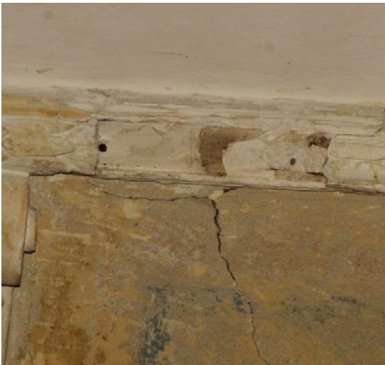
Fig. 7. Cracks on the surface of the vaults and loss of the molded ceiling decoration. Probe before the conservation, 2012. Photo by S. Hetmanchuk.
