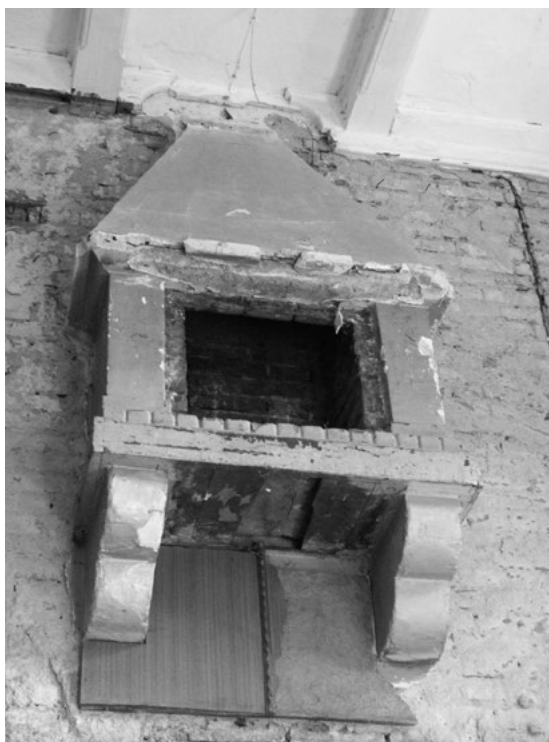
Fig. 7. Tatarów. "Straszny Dwór" guesthouse. Southern avant-corps , fireplace in the level of the first floor. Photo J. Czubiński, 2012.
