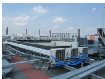
Fig. 14. Ventilation ducts (indicated with letter A in Fig. 13) on the roof of Renoma Department Store (photo by P. Kirschke).
