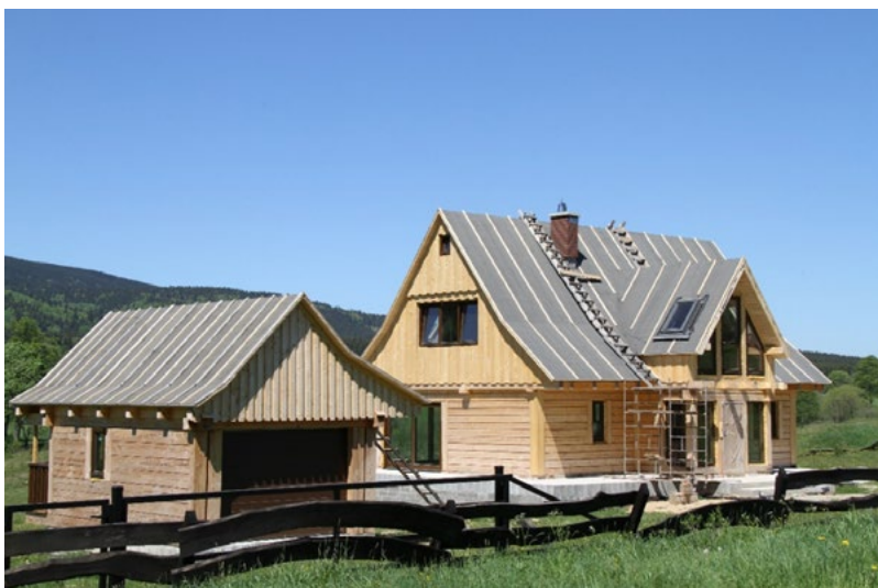
Fig. 24. Lasówka. A single-family building with a wooden structure and a garage under construction. It is a relatively successful attempt to refer in the architecture of the building to the regional heritage of the Kłodzko Land. Photo by the author. 2017.
