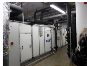
Fig. 16. The plant room (indicated with letter C in Fig. 13) located in the basement of Renoma Department Store (photo by P. Kirschke).
