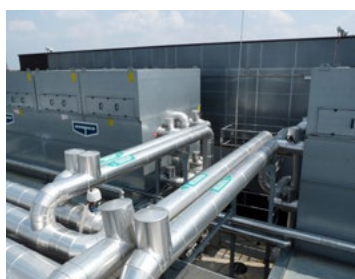
Fig. 15. Ventilation ducts (indicated with letter B in Fig. 13) on the roof of Renoma Department Store (photo by P. Kirschke).
