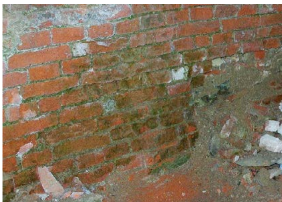
Fig. 24. Room No. 28. Deconsolidation of the top layer of bricks caused by chemical corrosion. Biological corrosion in the form of mosses and lichens.
