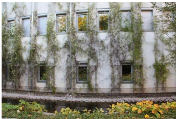
Fig. 5. The Opera and Philharmonic in Białystok – plants growing on the main hall. Photo: Andrzej Tokajuk.
