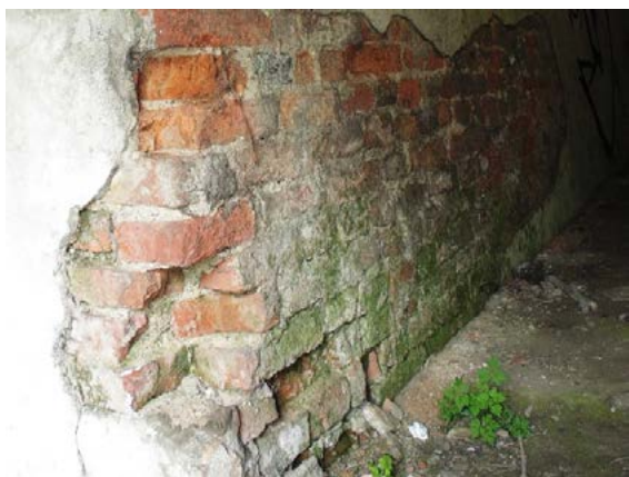
Fig. 21. Room No. 16. Losses of bricks in the structural wall and visible biological corrosion.
