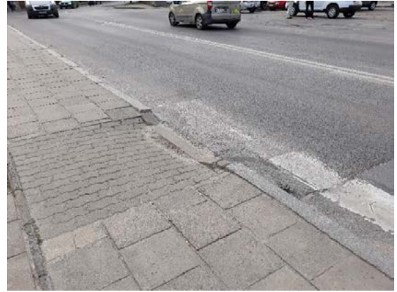
Fig. 14. Limited access to the zone of the pedestrian crossing, The Stefanidesa Square, Zamość. Photo: K. Kielin
