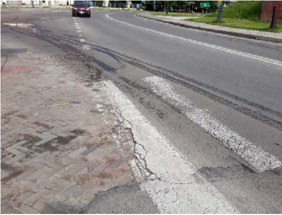
Fig. 13. The lack of pavement at the pedestrian crossing, The Stefanidesa Square, Zamość. Photo: K. Kielin
