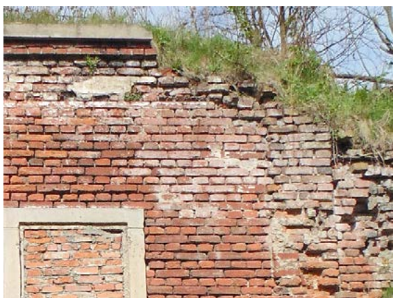
Fig. 13. The northern part of the Red Barracks. Significant damage to the corner of the front wall. Numerous cavities and shortages of bricks. Lack of joints.
