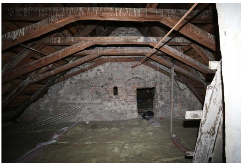
Fig. 10. The attic above the eastern annex of the monastery – a visible gable forming the gable wall of the monastery in 1569, photo by: K. Janus, 2012.
