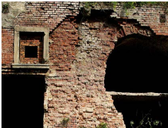
Fig. 16. The southern part of the Red Barracks. Extensive cavity in the front wall. South
