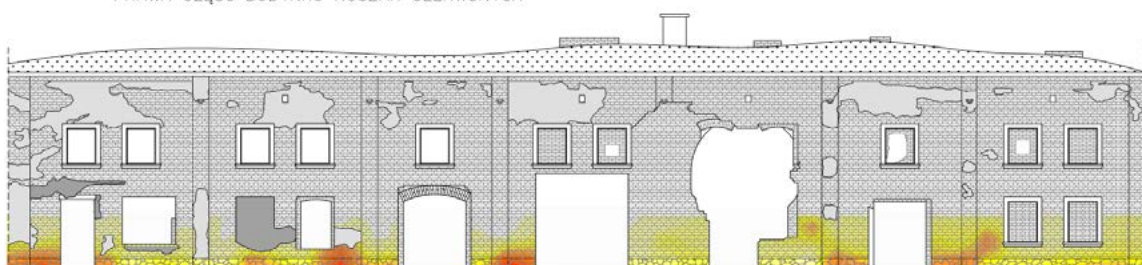
Fig. 10. Moisture map of the front elevation of the Red Barracks – southern part.
