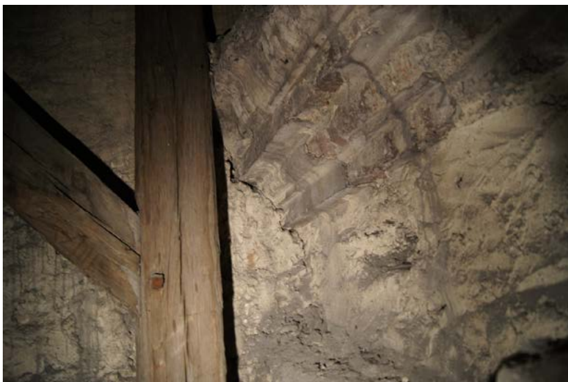
Fig. 3. The level of the attic above the southern nave of the Bernardine church, view of the cornice of the original façade, made between 1557 and 1569, photo: K. Janus, 2012.
