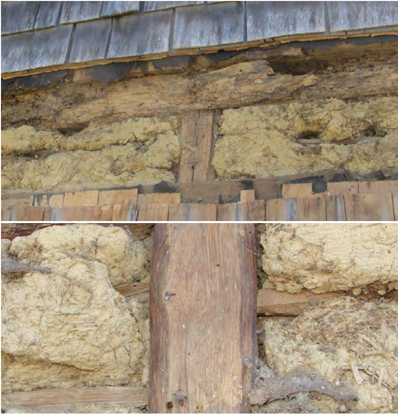
Fig. 5. Top: Clay and straw infill in the exterior wall of the Hancock-Mitchell House, Chilmark, Massachusetts (Myron O. Stachiw, 2015)
