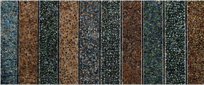
Fig. 13. Detail of the glass mosaic on the façade of the “Cepelia” exhibition pavilions in Częstochowa by Włodzimierz Ściegienny, present state. (photo by H. Wąsek).
